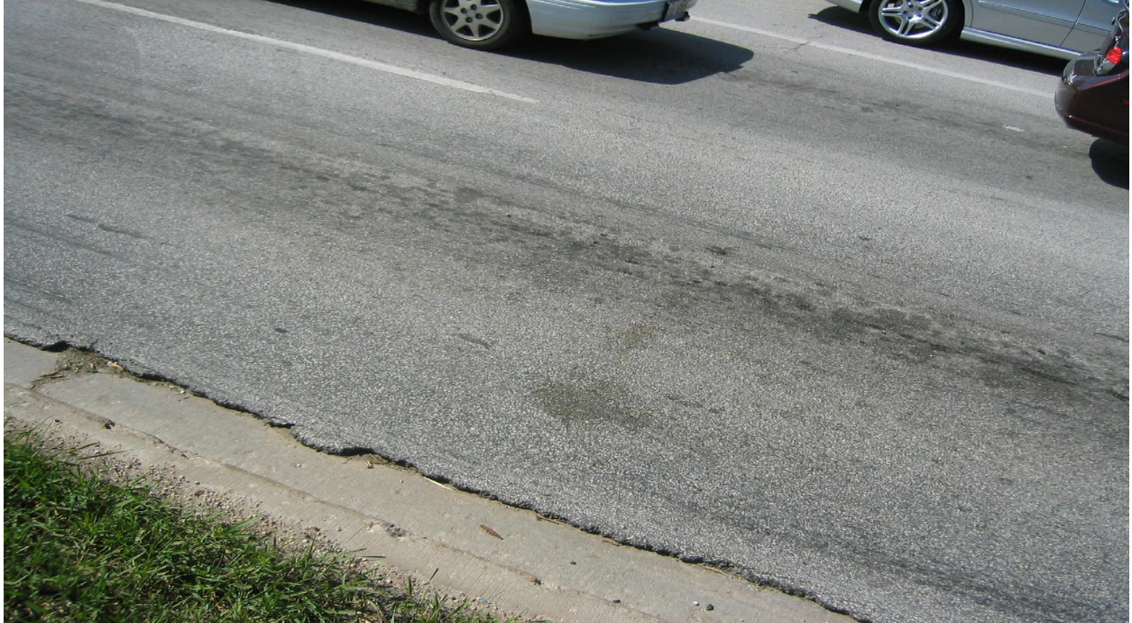
Severe Rutting on Fabyan Parkway near the Eastbound Stopbar
